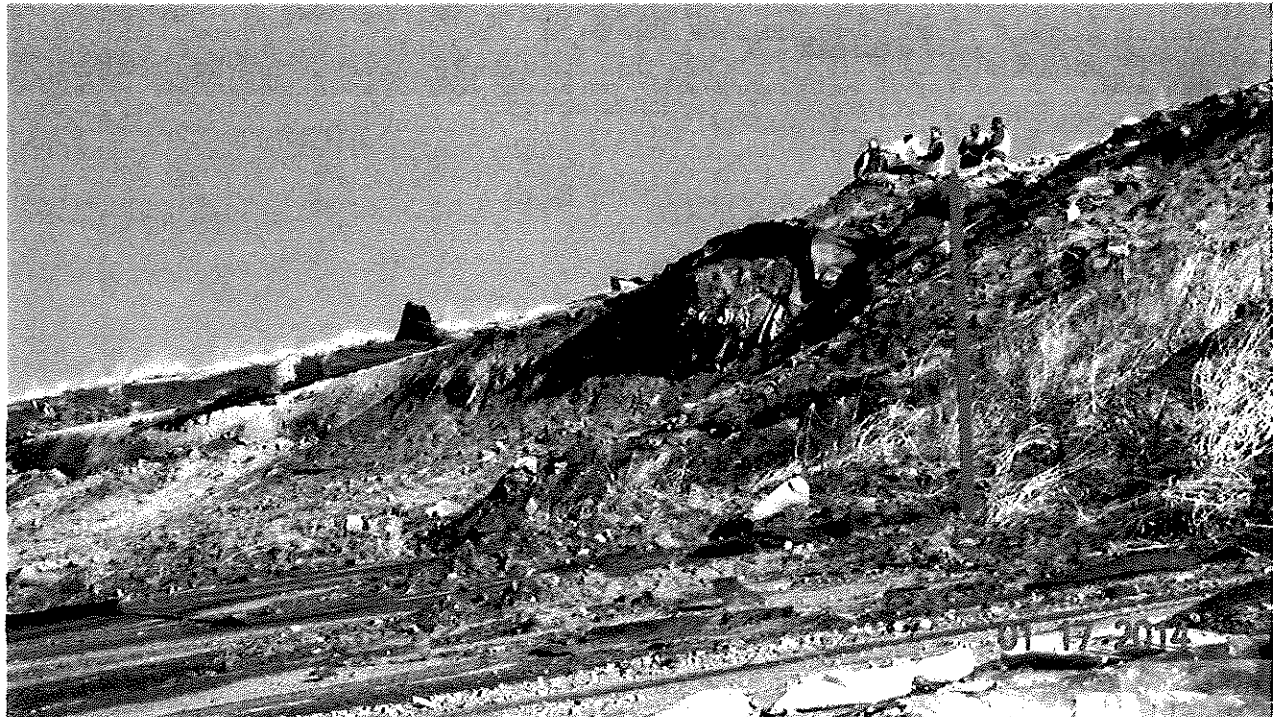
Figure B-12: Close-up of exposed waste and cover soil at top of slope (see red arrow) where failure surface exited the bottom liner system and passed through the waste.
