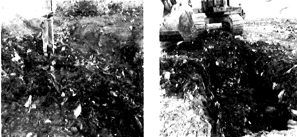
Figure B-20: Excavations in waste to measure moisture content and unit weight.
